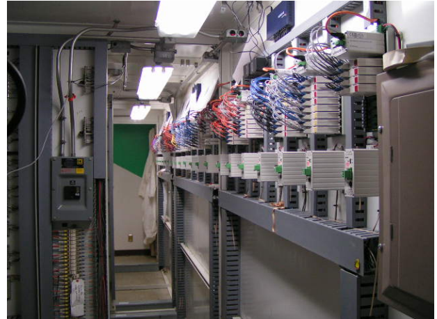
More than 2500 Opto 22 SNAP PAC System I/O points monitor and control water treatment processes around the clock
