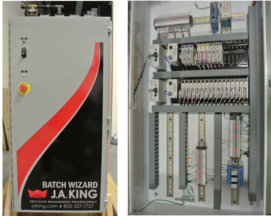
J.A. King I/O cabinet for automated ingredient batching Exterior (left) and interior (right), with Opto 22 Ethernet I/O
