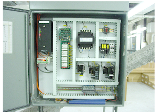
One of the many roof monitoring panels using Opto 22 G4 I/O with SNAP-LCSX Controllers
