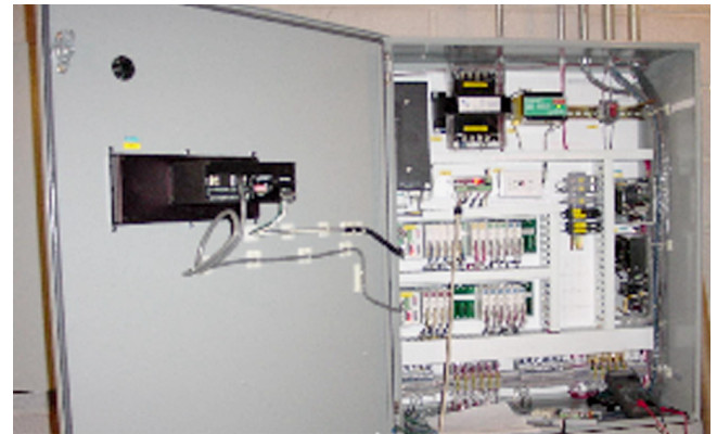
Domestic hot water control panel outfitted with Opto 22 SNAP controllers and I/O system
