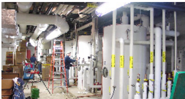
The photos above show one of the numerous mechanical rooms with hot water plumbing systems. This system is controlled by the domestic hot water control panel.
