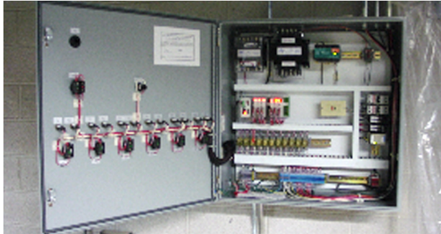
Remote waste cutoff control panel with pit level control
