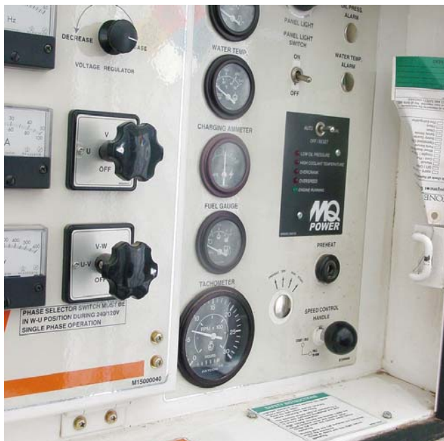
Figure 2: Control and Monitoring Gauges Inside the Generator Housing
