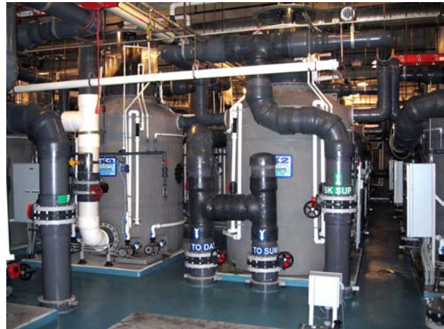
Water reclamation tanks
