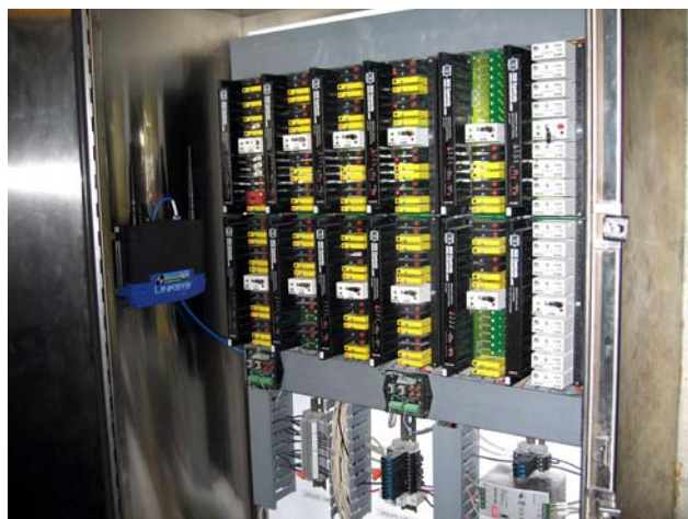
Opto 22 I/O in a Georgia Aquarium control panel. A Linksys router provides wireless connectivity.
