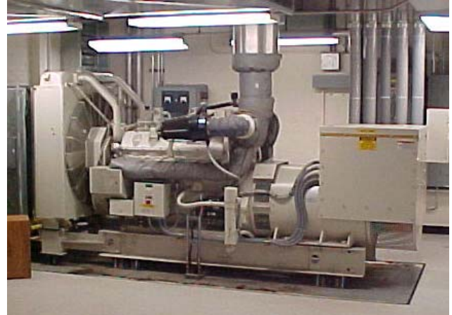
Opto 22 remote monitoring systems monitor Verizon generator sets.
