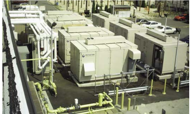
Seven fuel cells provide power to the Garden City CO.
