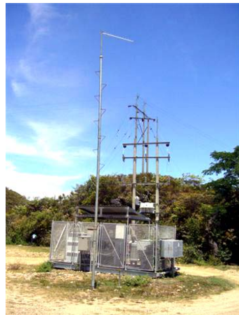
SINCRON established a wireless Ethernet network at each pumping location for transmitting operational data back to Ecopetrol headquarters.
