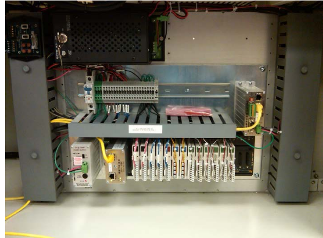
Advanced Energy's furnace I/O upgrade utilized the SNAP-PAC-EB1 brain.
