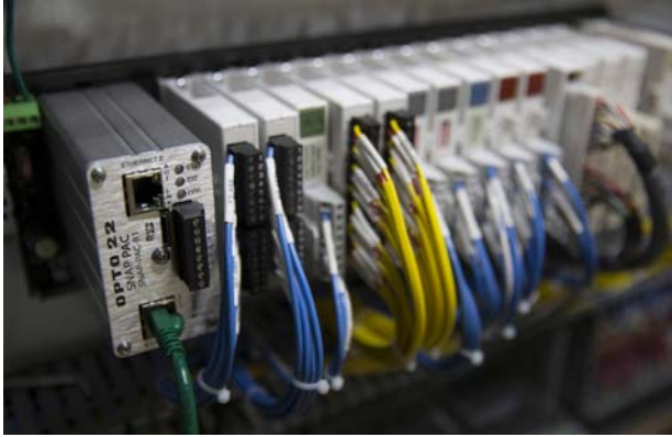
Opto 22 PAC controllers and SNAP I/O modules are used to monitor and control all processes.
