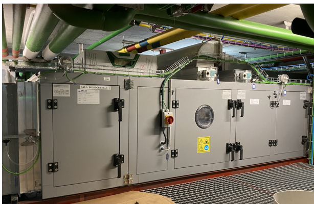
Air Handling Units (AHU) guarantee sterile conditions inside production areas.
