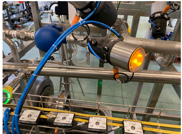
groov EPIC also integrates the Water for Injectables (WFI) plant using ASi bus.
