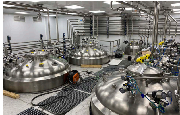
Fill and Finish Tanks during commissioning
