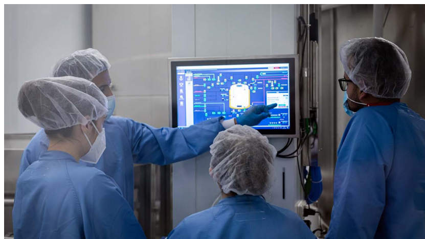
Touchscreens installed inside sterile areas allow operational staff to interact with the system. [Photo credit: Cristina Galán]
