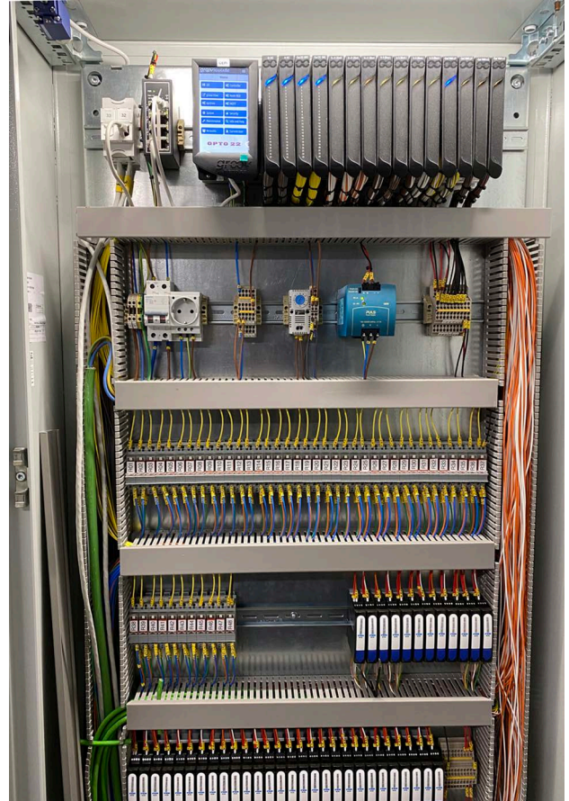
One of the many groov EPIC distributed control system cabinets
