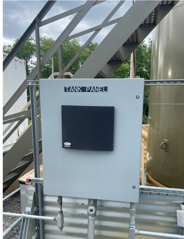
Pad control panel
