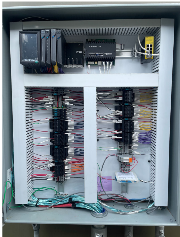
The groov EPIC (upper left) controls the well pad
