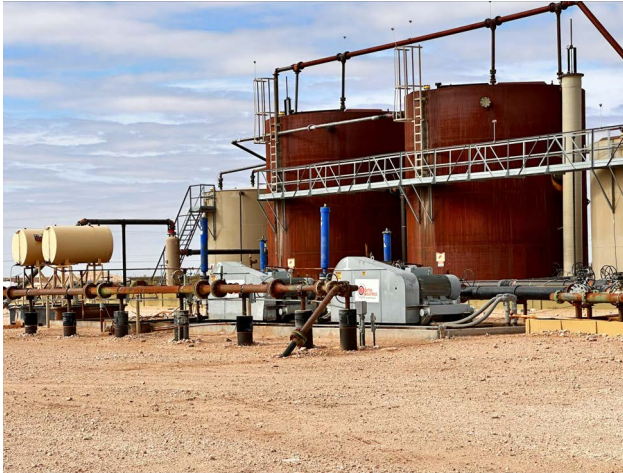
Point Energy Partners pump equipment at SWD site
