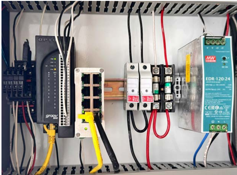
Point Energy Partners' groov RIO enclosure
