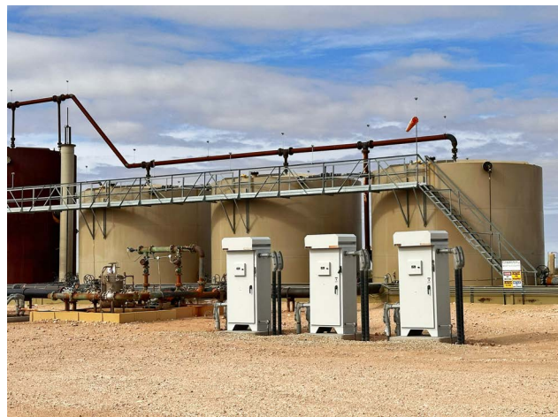
Tanks at Point Energy Partners SWD site
