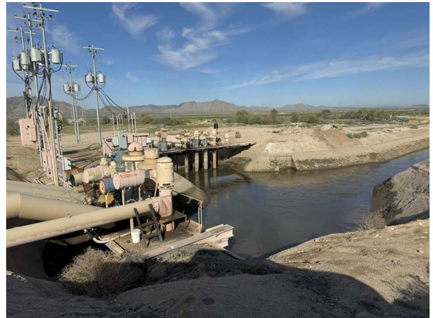
Paloma Irrigation lift station
