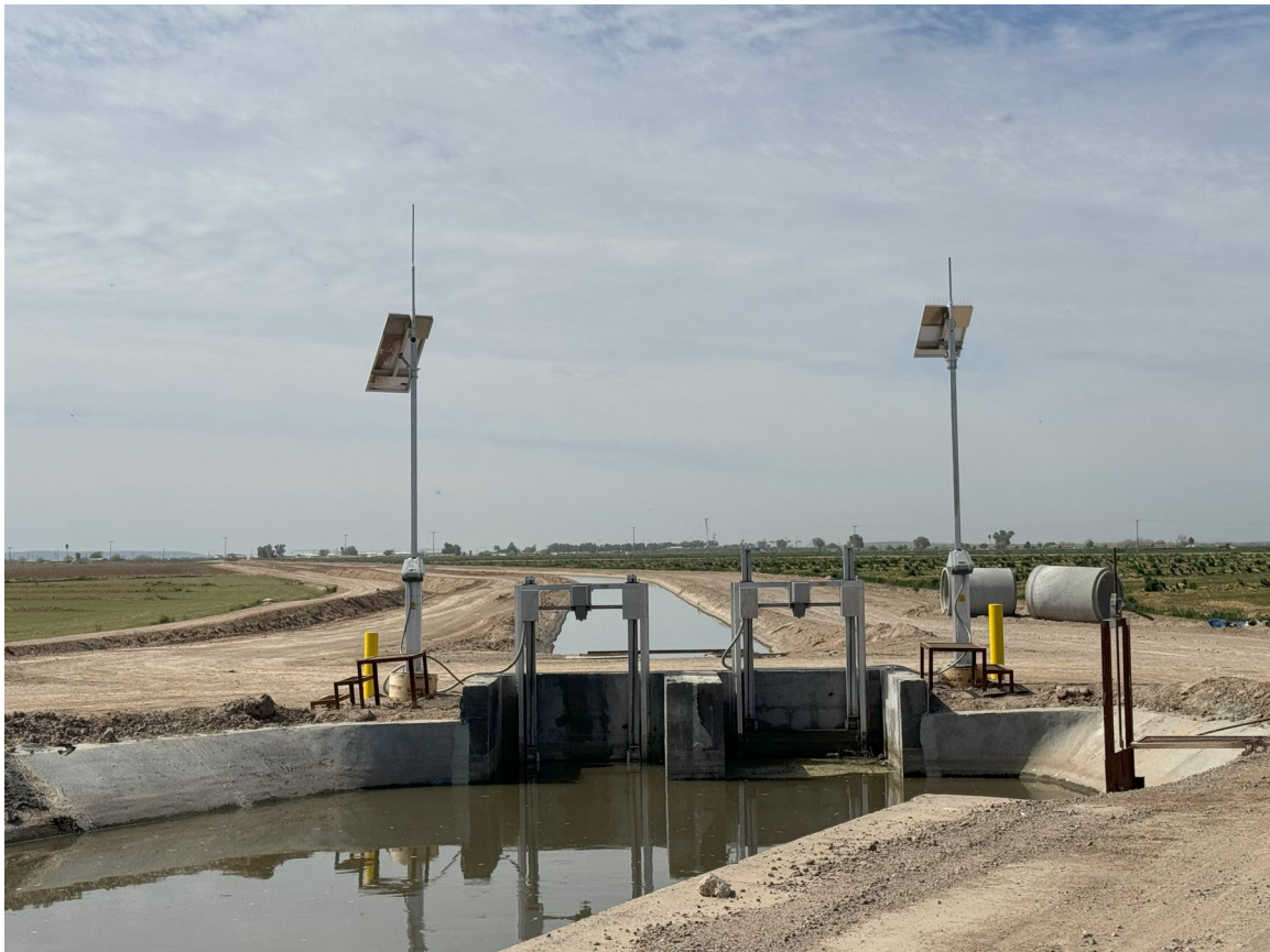
PIDD solar-powered, automated control gates
