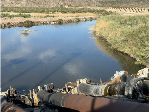
Gillespie Dam lift pumps
