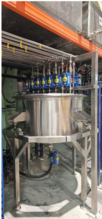
Dosing hopper at Pinturas Tropical
