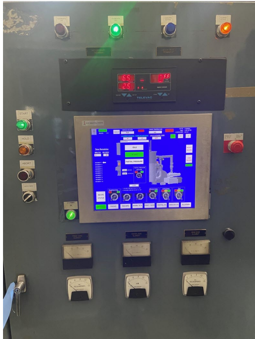
An easily accessible HMI monitor of the Mercer equipment layout
