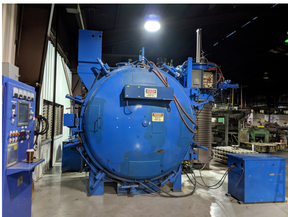
Vacuum furnace (exterior)
