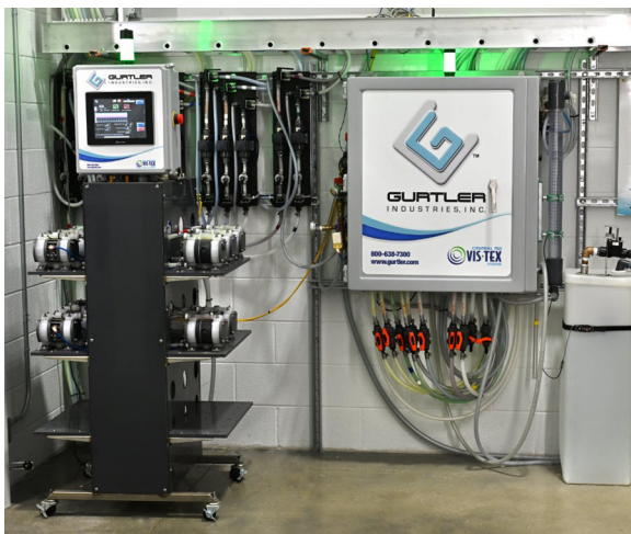
The control panel and dispensing pump from Gurtler Industries
