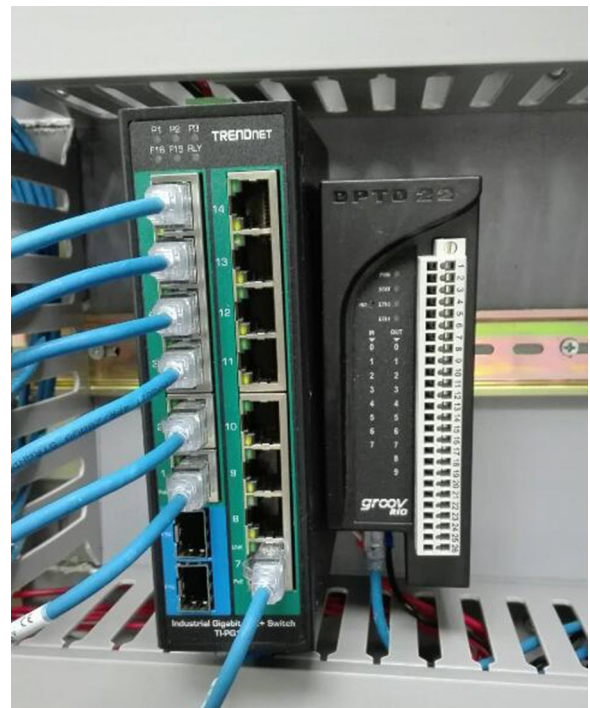
groov RIO and network switch inside the MVRES electrical panel
