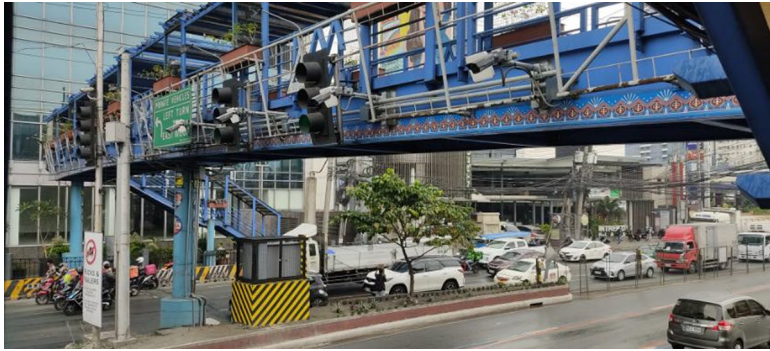
Each IDF substation is equipped with IP cameras and RFID readers.
