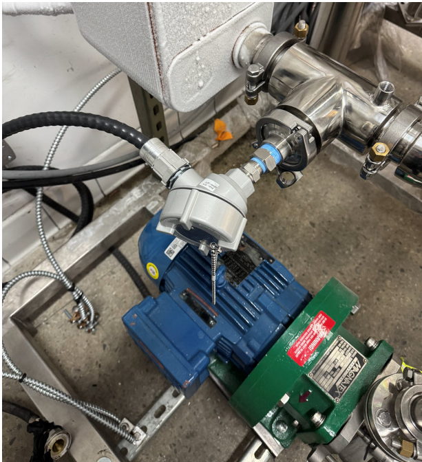
PermaCool's process plumbing shows insulated lines and mounted precision temperature sensors for accurate feedback control
