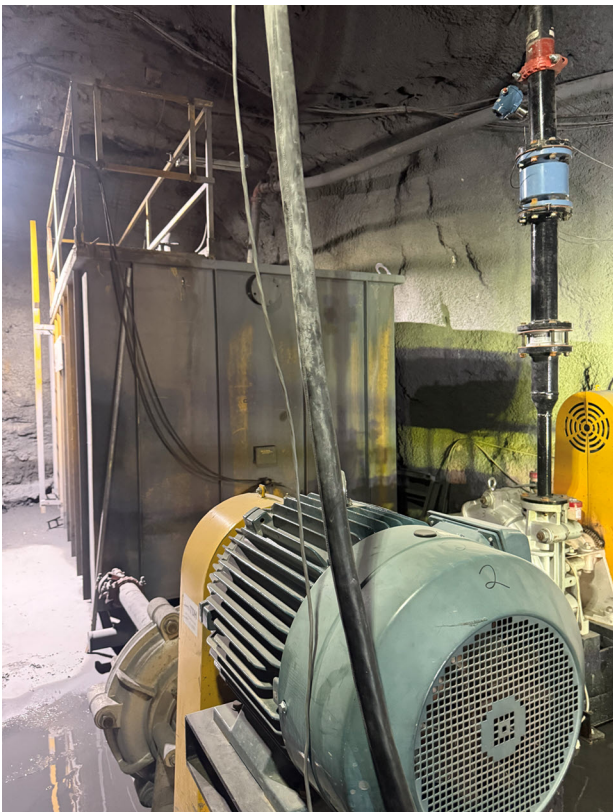
A sump pump motor and tank in an underground pump station
