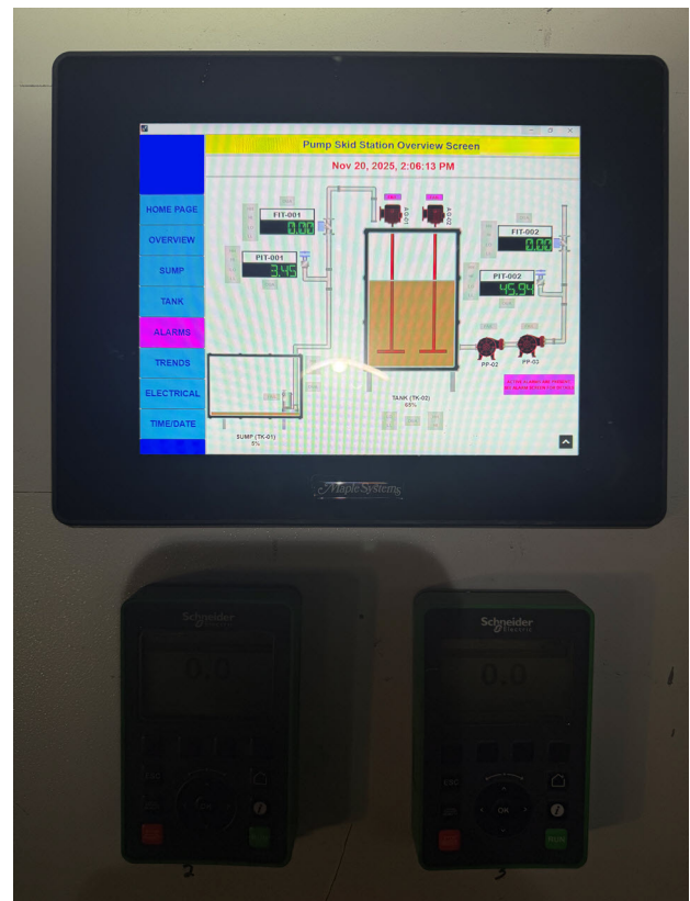
Visualization through an easily accessible HMI screen outside of the control panel
