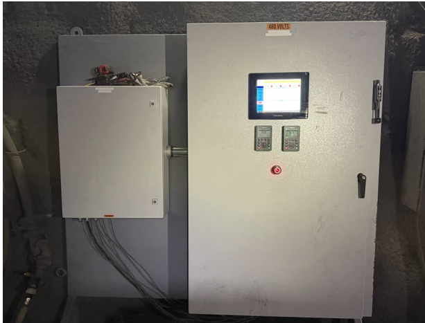
The new sump control panel runs Ignition for pump monitoring and control.
