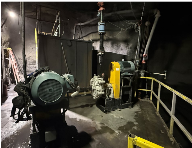
The upgraded underground sump pump station with dual slurry pumps and tank
