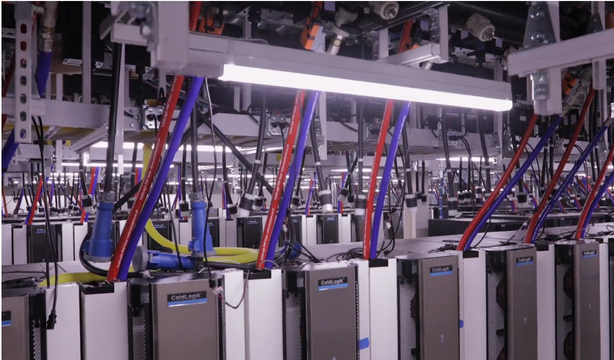
Rows of servers are cooled by rear-door heat exchangers connected to the barge's river-water cooling system.
