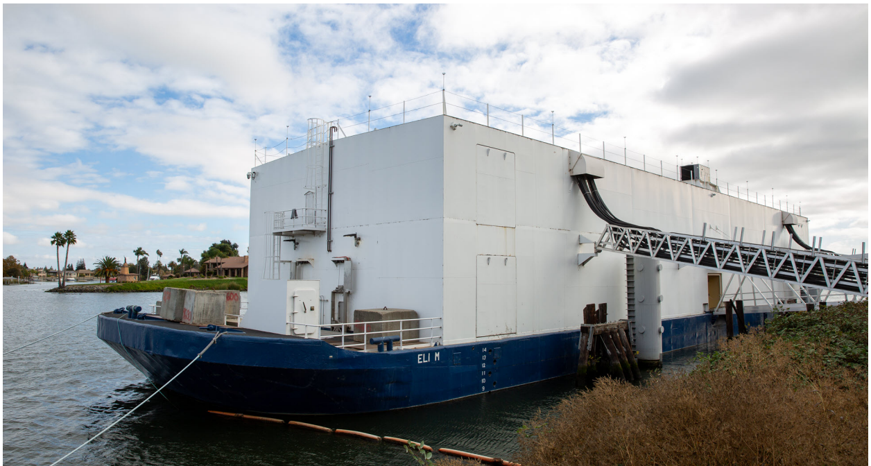
Nautilus Data Technologies' first liquid-cooled data center sits on the San Joaquín River in Stockton, CA.
