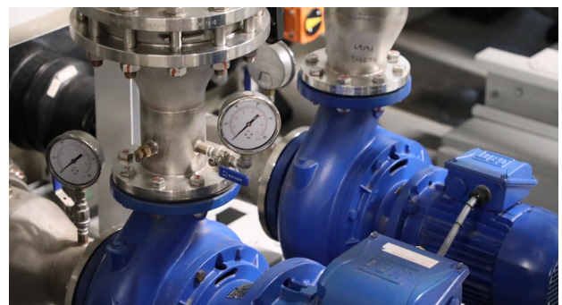
Measuring pump discharge pressure to monitor system performance
