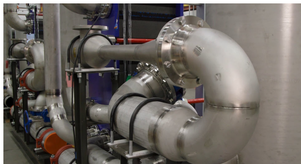
Heat exchangers transfer heat from the data center cooling loop to river water.
