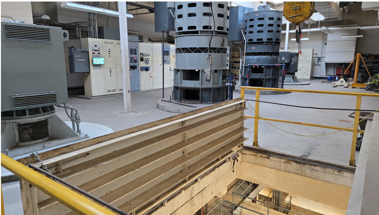
Legacy systems in remote water and wastewater stations operated reliably with established controls, but using legacy communication methods made system-wide visibility difficult.
