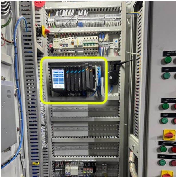
The control panel was built around a groov EPIC processor, with cellular backhaul and field wiring to pumps, blowers, and sensors.
