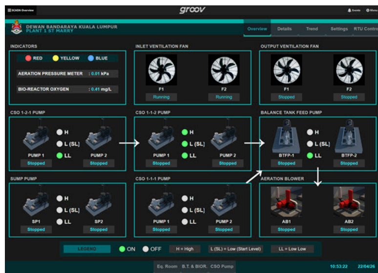
The St. Mary plant overview in groov View shows CSO pumps, balance tank, bioreactor, blowers, and ventilation status on one screen.
